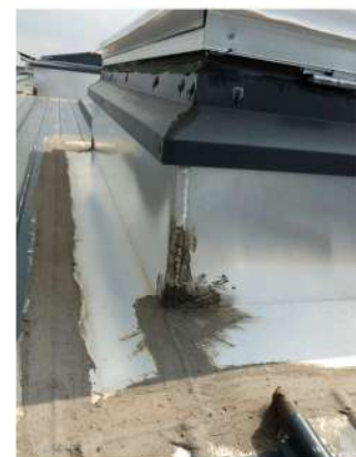
PHOTOGRAPHIES OF THE ZONES WITH WATER STAGNATION
