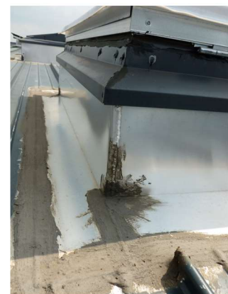
PHOTOGRAPHIES OF THE ZONES WITH WATER STAGNATION
